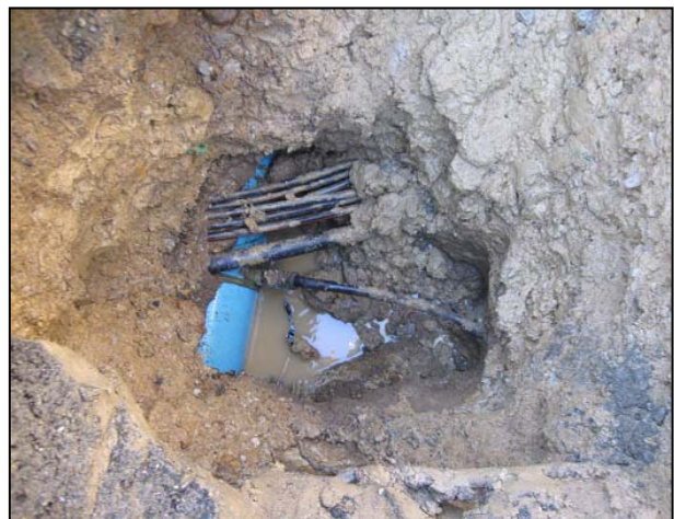
Where SMUD Power & AT&T lines actually were, directly on top of our water line.
