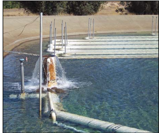
Tertiary Recycled Water flowing into the Equalization basin before delivery to the RMCC.
