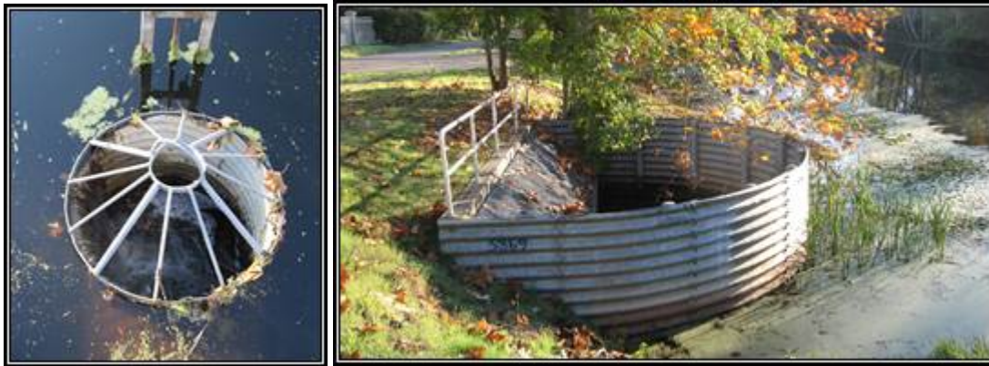
photo of the inlet to Low Flow outlet & High Flow Outlet
