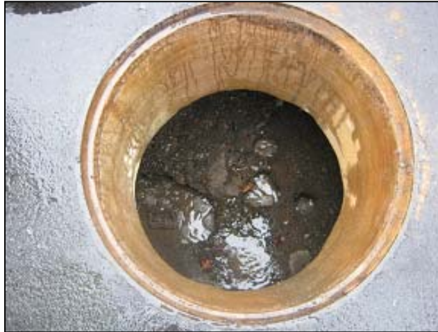
Storm drain on Reynosa Dr. filled with sand and debris prior to cleaning by staff
