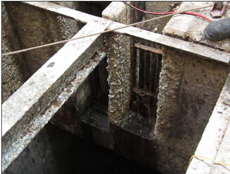
Concrete corrosion leaving aggregate used in concrete exposed as well as damaging aluminum beams used in decking support.
