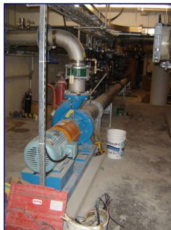
Figure 3.12: New pumps in filter gallery
