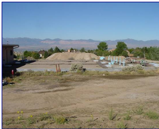
Figure 3.2: Photographs of the Draper, UT 6.6 MGD WTP
