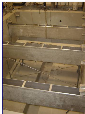
Figure 3.10: New membrane tank
