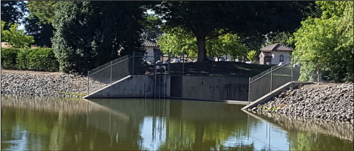
Photo of Spillway at Laguna Joaquin with staff gauge and drain valve on left side
