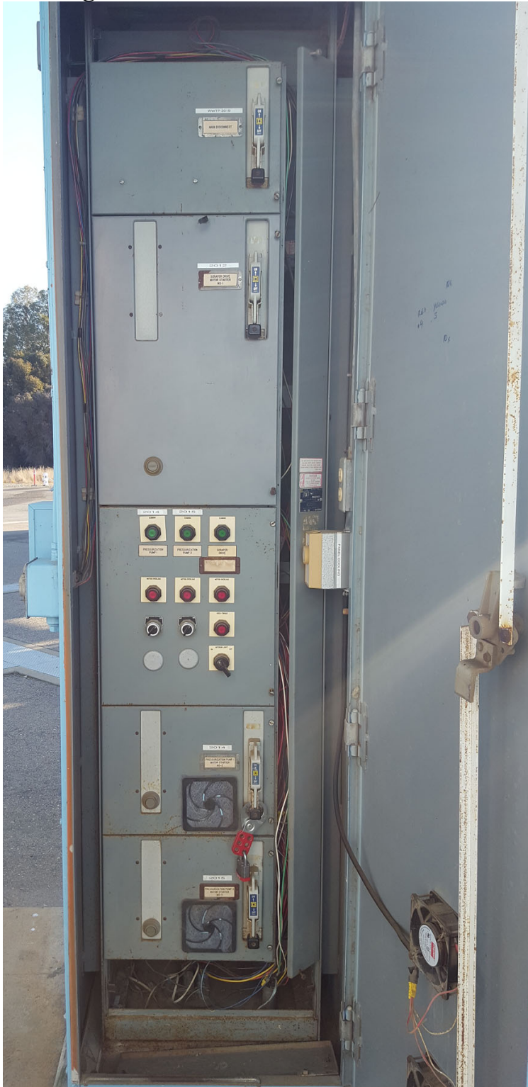
Existing West DAF cabinet – Outside view
