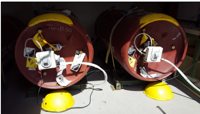
Existing Chlorine tons and feed system
