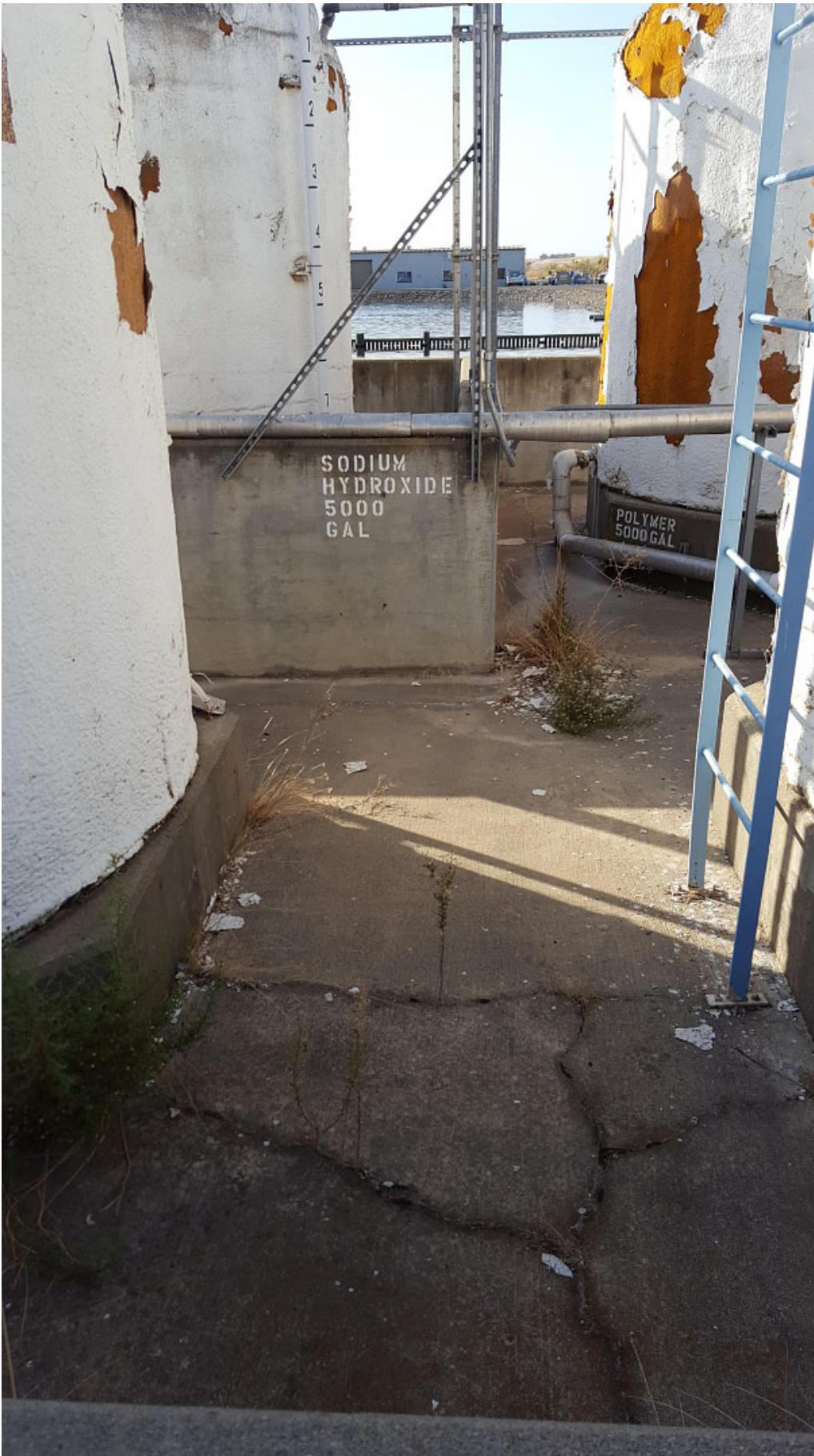
View from existing acid tank in left foreground and caustic tank in background
