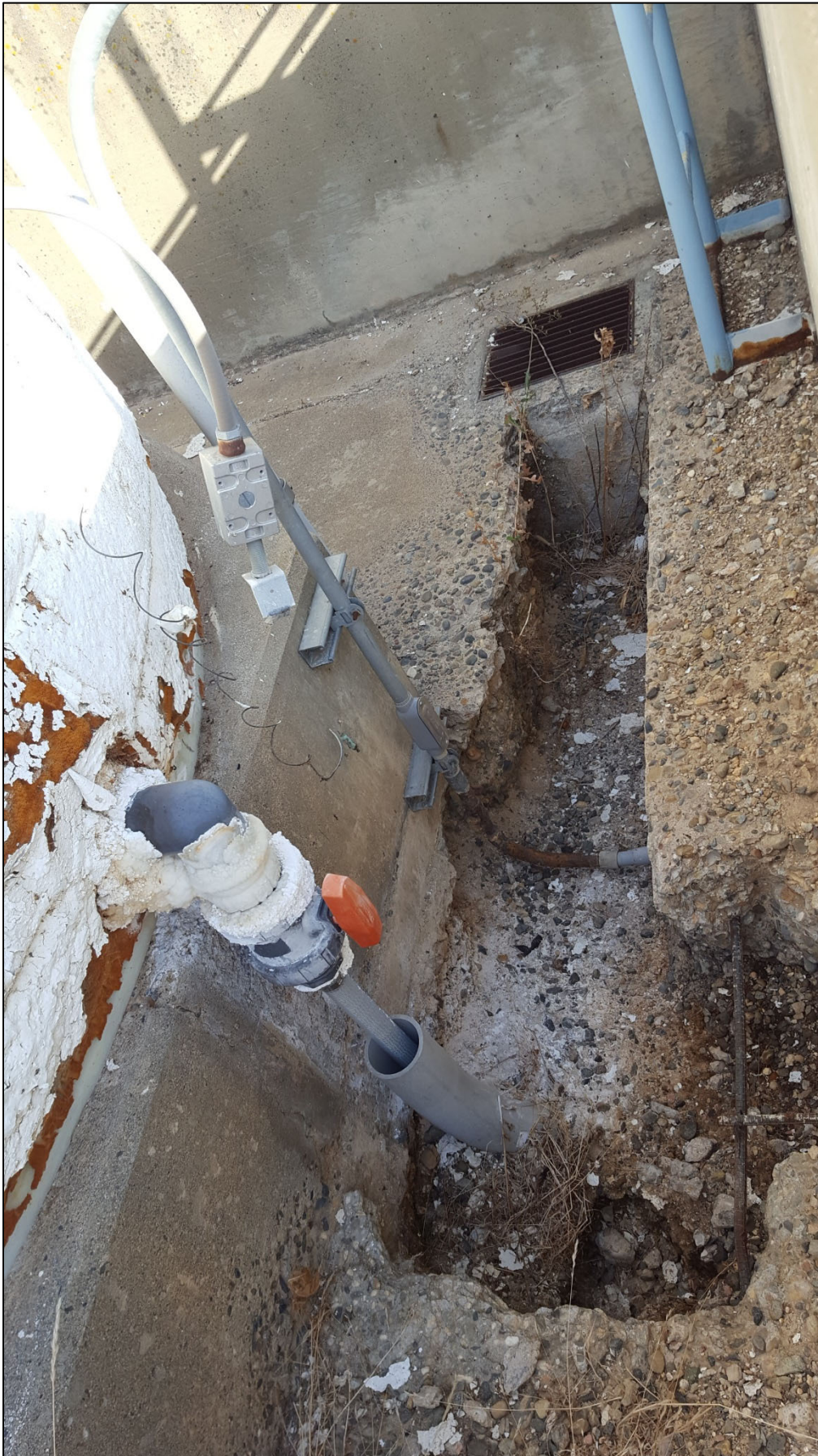
View of discharge from existing caustic tank
