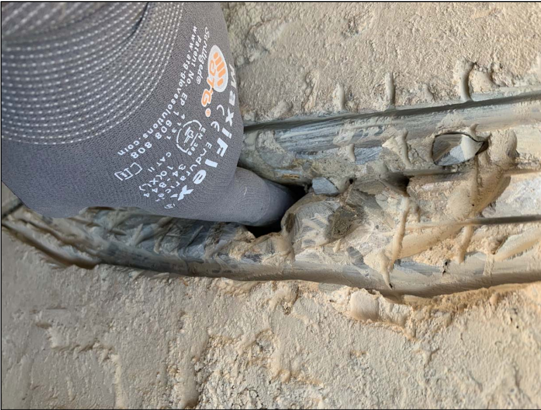
Hole in CIA diversion box next to Country Store, prepped for repair
