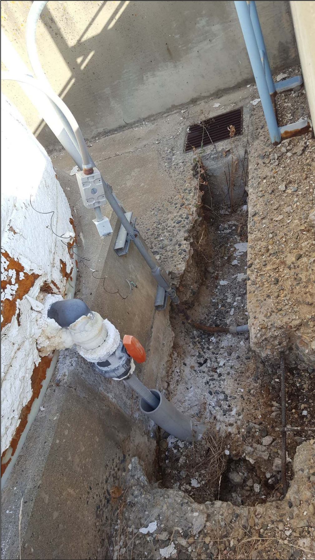
View of discharge from existing caustic tank
