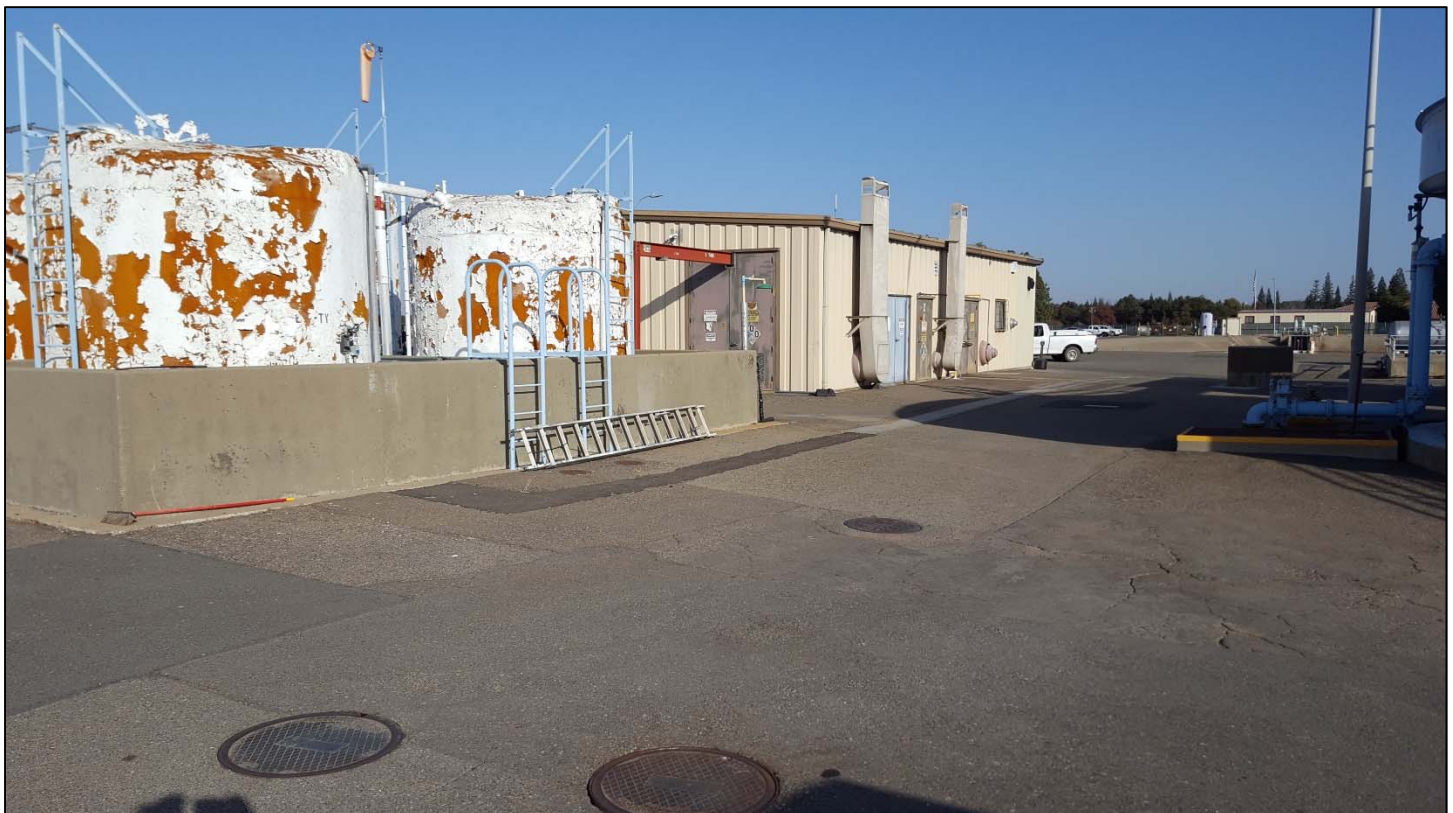
View of bulk chemical tanks, trench, and control building at tertiary treatment facility
