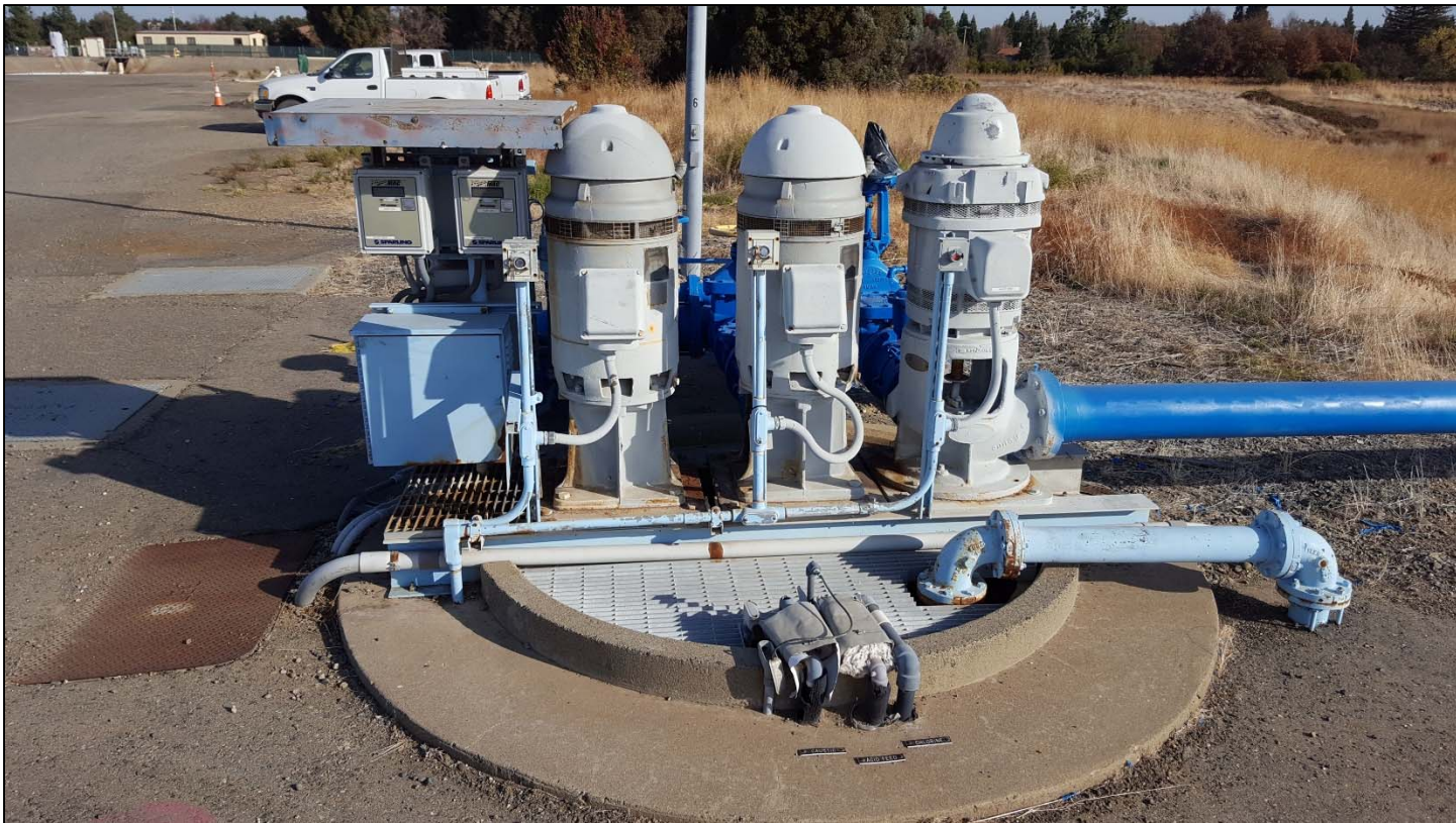
Tertiary pump station with chemical feed lines feeding into wet well
