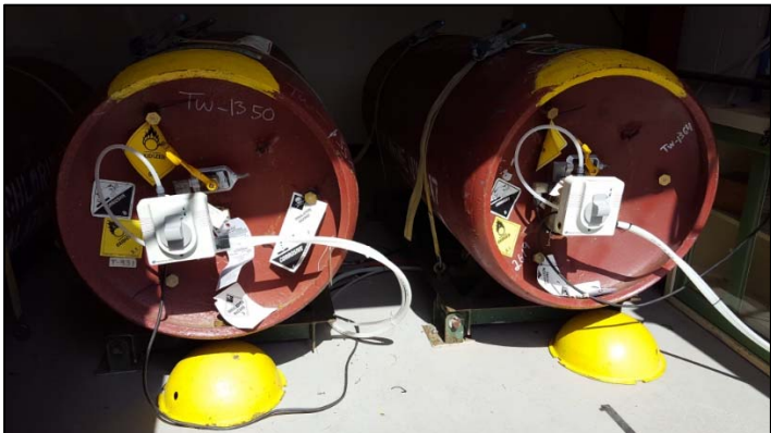
Existing Chlorine tons and feed system
