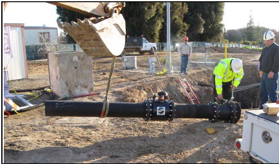
Staff installing a new magnetic flow meter for the North Course Pump Station discharge.
