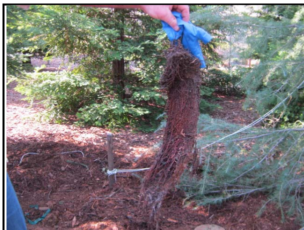
Redwood tree roots removed from a private sewer lateral.
