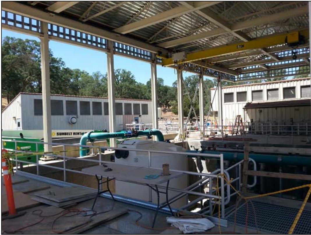
View of CIP tank
