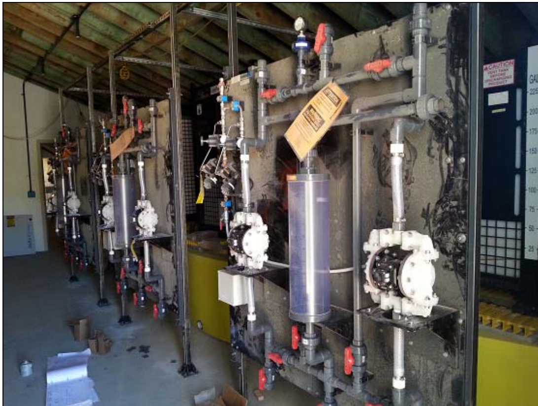
Chemical feed equipment and storage tote behind them
