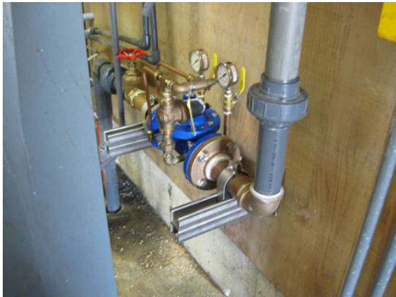
New pressure reducing valve installed at Water Plant.
