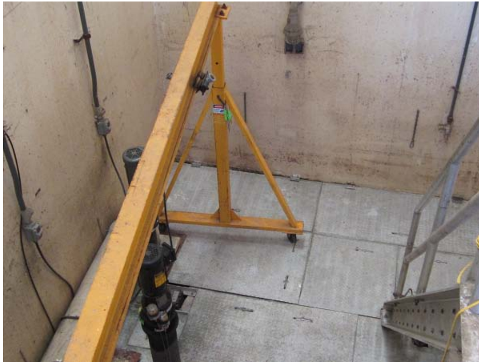
Interior view of wet well side of MLN showing comminutors and stairway they have to be pulled up on for servicing.
