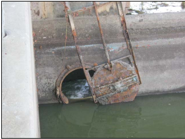
Photos of corrosion damage on old slide gate valve at Laguna Joaquin
