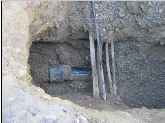
Sewer line damage on Pera Drive (before)
