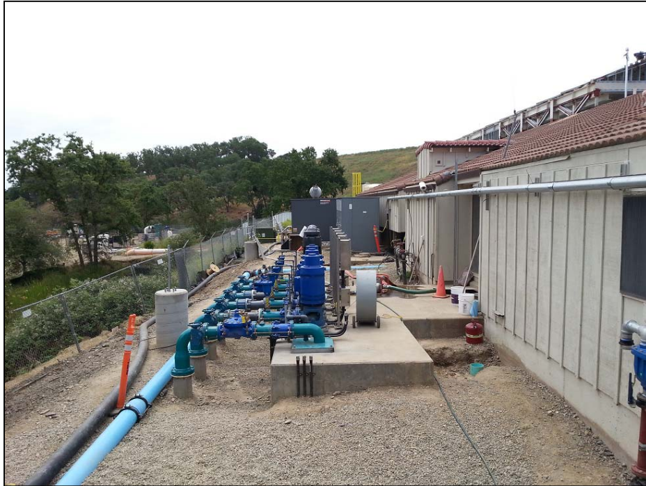
Effluent Pump station
