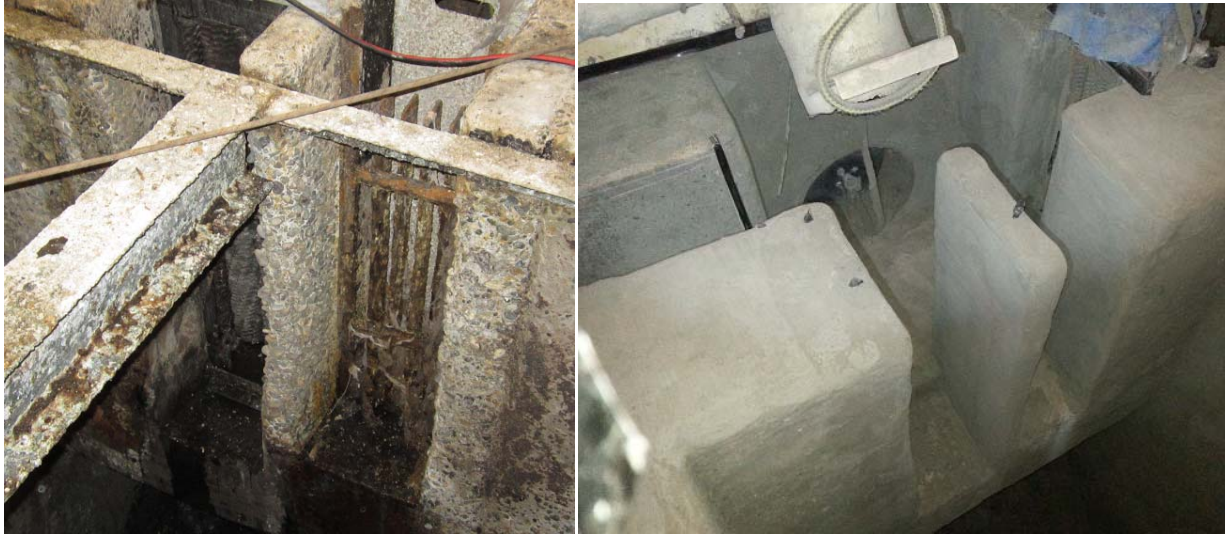
Influent channel of Main Lift North sewer pumping station, before and after being repaired with Quadex Aluminaliner
