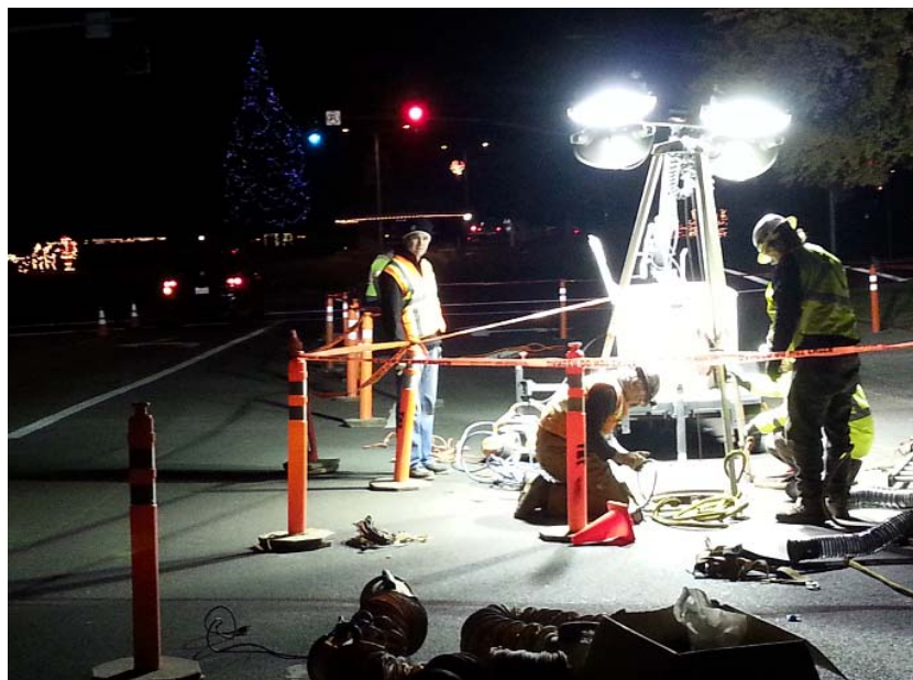
Standing by at 1:30am while TNT attempted to install a flow-through bypass 12/20/13 in manhole near Country Store
