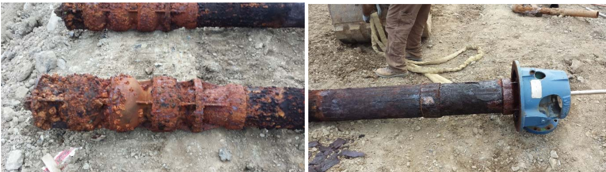
Photo of one of the pumps taken 3 years ago showing advanced corrosion
