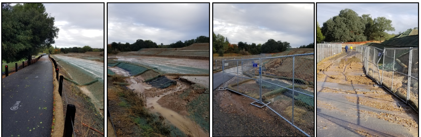
Post Storm pictures 10/25/2021
