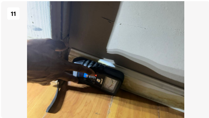
Baseboard moisture reading
