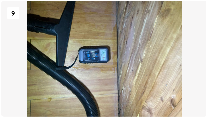
Moisture reading of wood and second area in hallway
