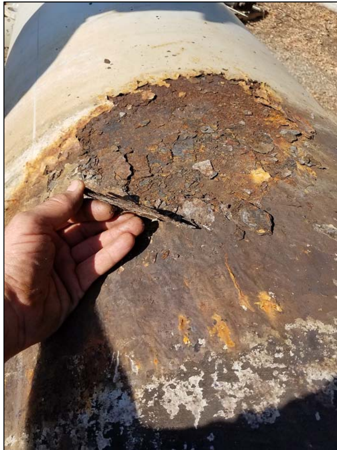
Corrosion of pipe column
