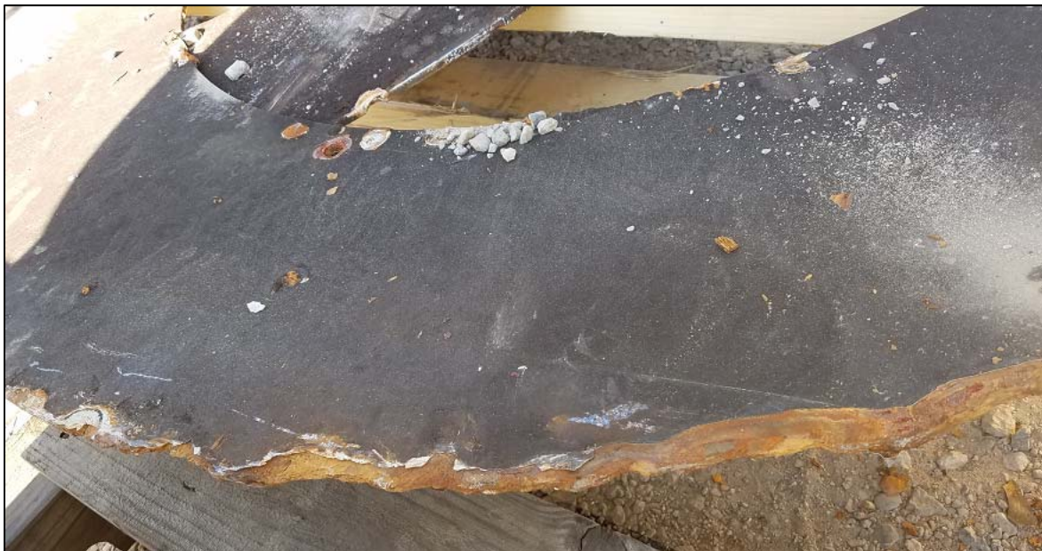
Corrosion of Vortex Plate of pump 2
