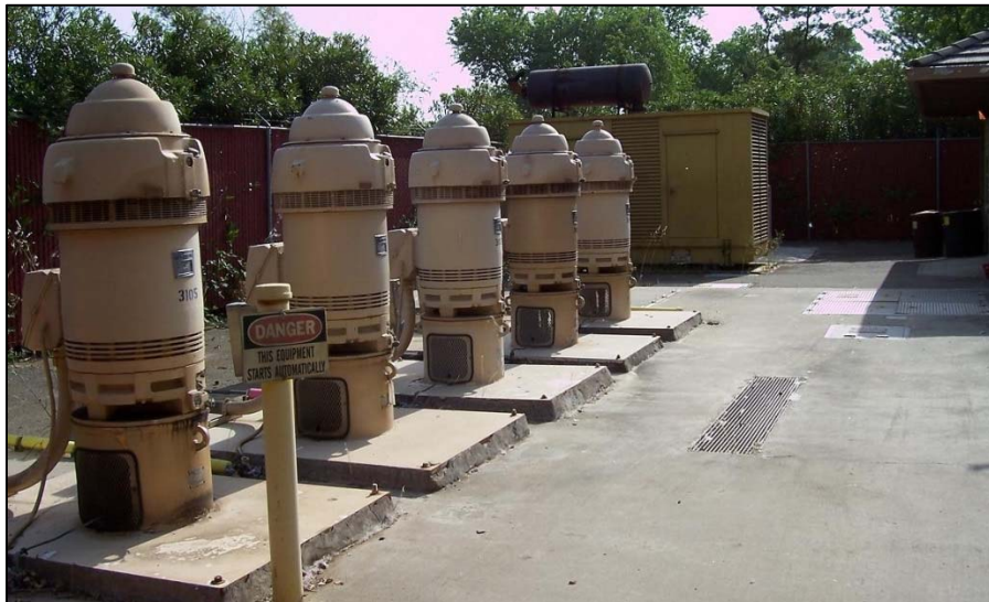
MLS Stormwater Motors, pumps are located beneath the motors.
