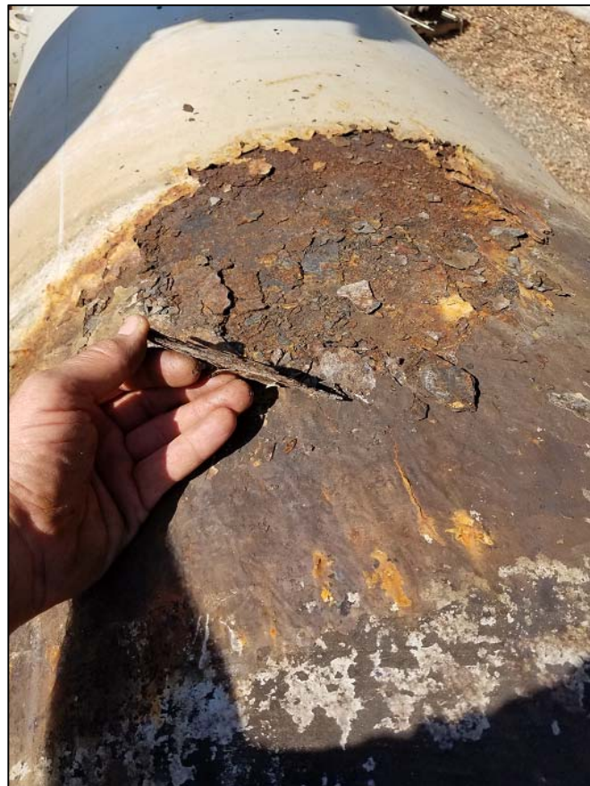
Corrosion of pipe column
