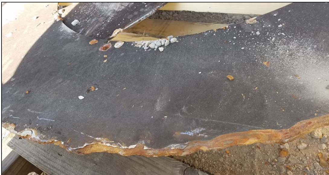
Corrosion of Vortex Plate of pump 2
