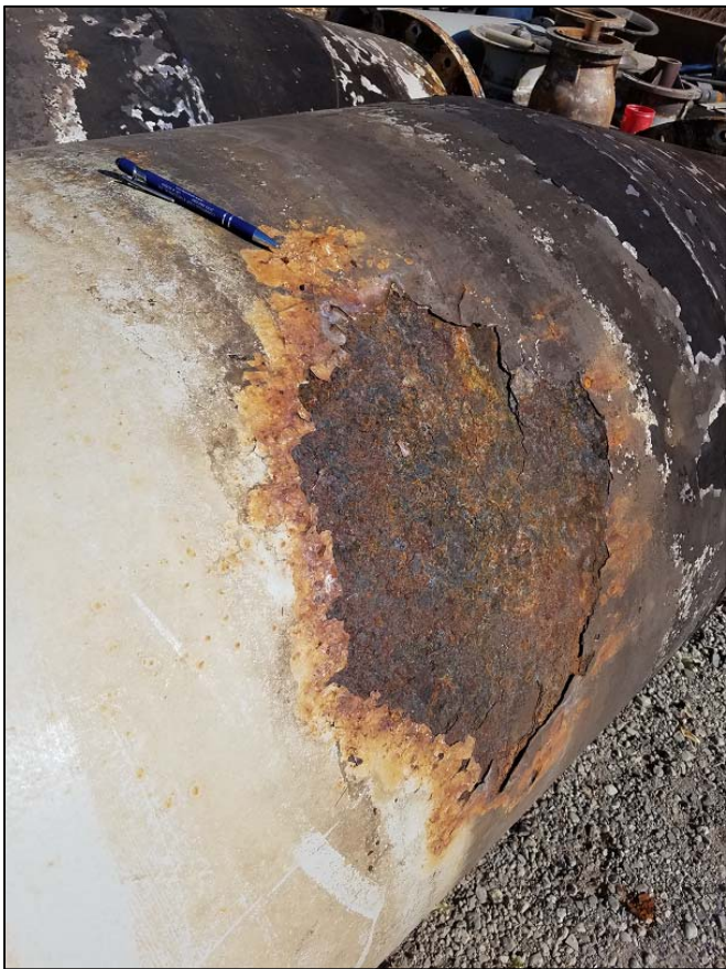
Corrosion of pipe column
