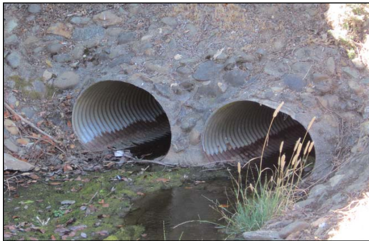
Entrance to existing Hole 13 North culvert pipes showing bottoms rusted out.
