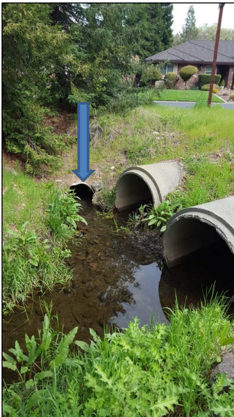
Outlet pipe from Zieour drainage
