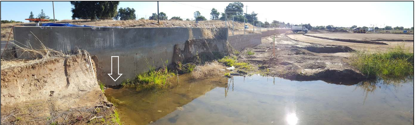
Photo of Cosumnes Irrigation Association diversion box next to Country Store with water leaking out from it and running into drainage with arrow indicating point of leak.
