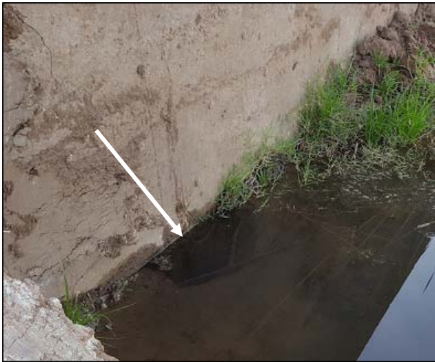
Closeup view of visible point of leak from CIA diversion box
