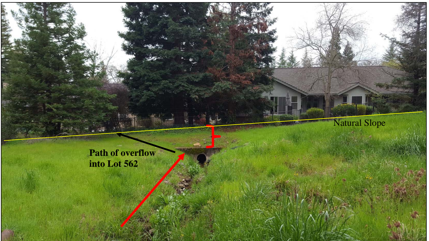
Photo marked up with flow path, natural slope, and area above pipe headwall
