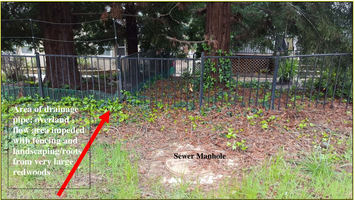
View looking down between Zieour Lot 562 (left) and Lot 560 (right); red arrow indicating path of drainage pipe and ideally where overland flow path should probably be.
