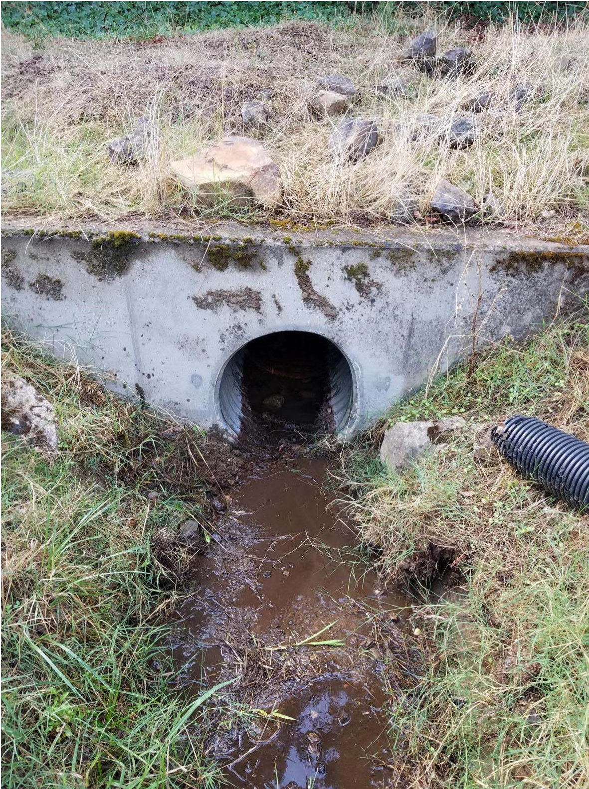
Up close photo of pipe entrance
