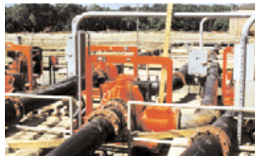
Wastewater Treatment Plant Bypass Project – Temporary installation of twelve 12" (300mm) DPC300 electric drive Dri-Prime pumps
