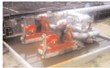
API Separator Sludge Removal – Permanent installation of two 6" (150mm) CD150M electric drive Dri-Prime pumps
