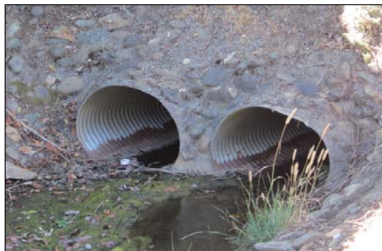
Photo of entrance to existing Hole 13 North culvert pipes showing bottoms rusted out.
