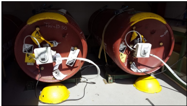
Ton cylinders of chlorine gas
