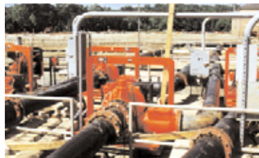
Wastewater Treatment Plant Bypass Project – Temporary installation of twelve 12" (300mm) DPC300 electric drive Dri-Prime pumps
