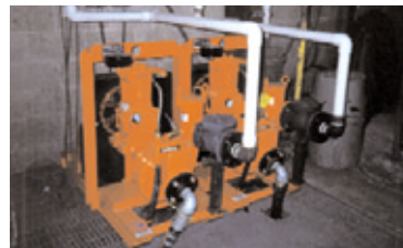
Industrial Wastewater Management – Permanent installation of two 3" (75mm) CD80M electric drive Dri-Prime pumps
