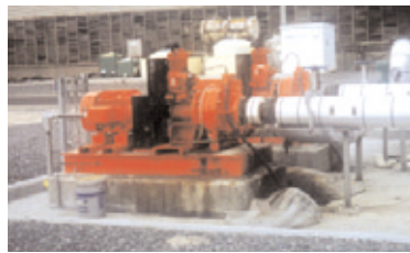
Industrial Storm Water Sump – Permanent installation of two 6" (150mm) HL5M electric drive Dri-Prime pumps
