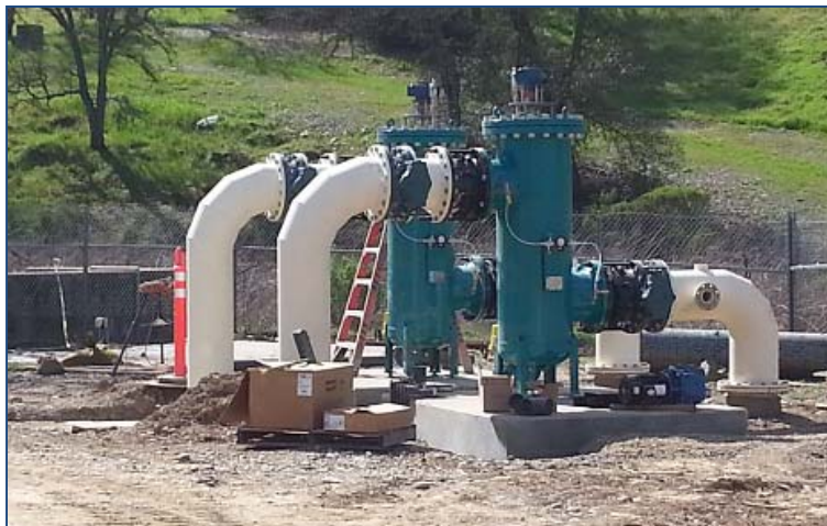
Raw water automated screening system
