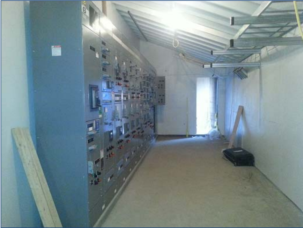
Motor Control Center for Plant#1
