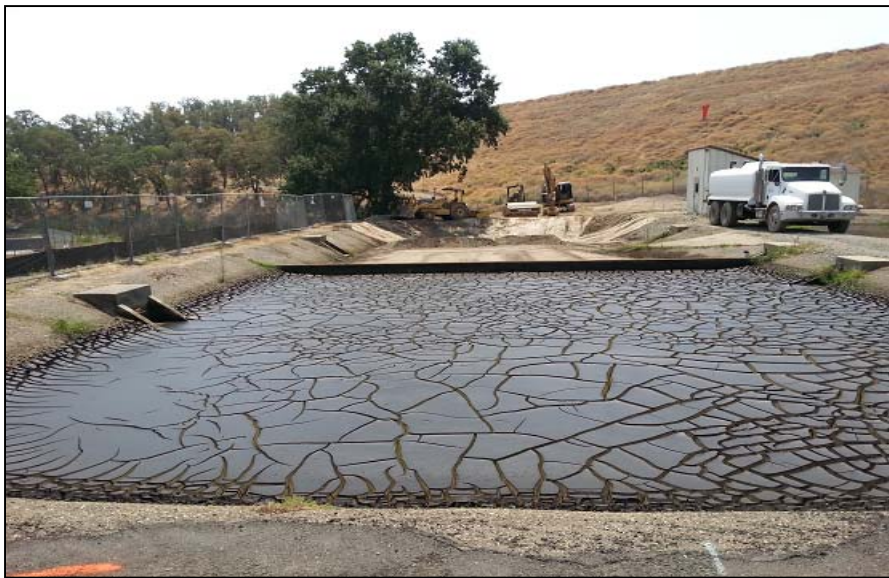
Backwash solids drying bed extension work in background, existing drying bed in service in foreground.
