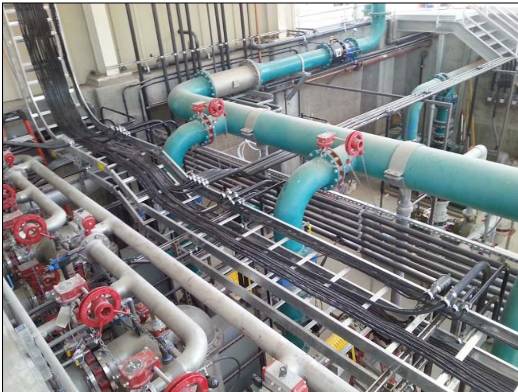
View of power and control system wiring, air lines, and permeate discharge piping.
