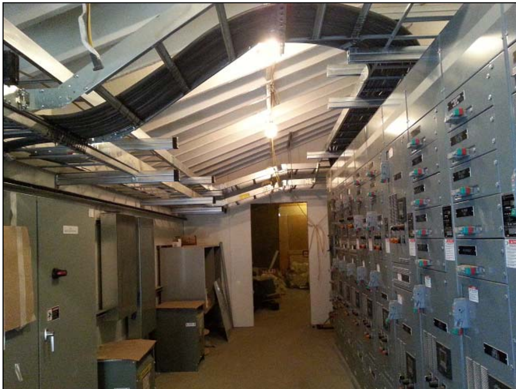
Membrane motor control center
