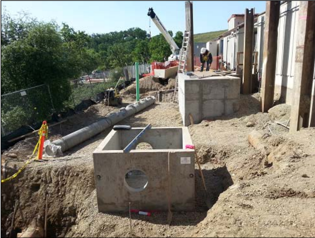
Effluent meter vault in foreground and completed Effluent Pump station in background
