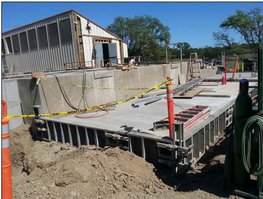
Concrete pads for Plate Settler in foreground and Neutralization tank in background
