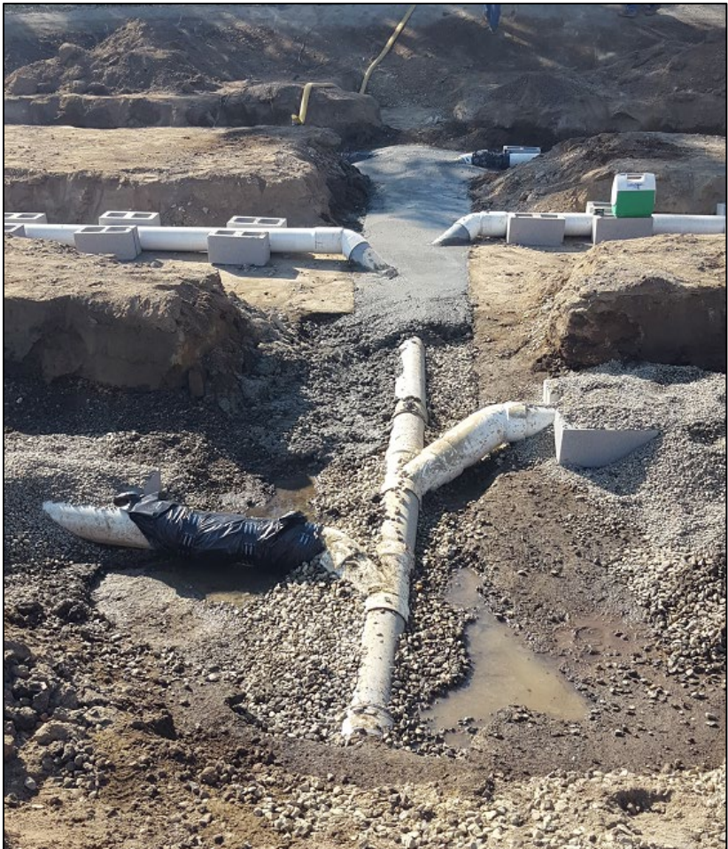
New piping layout before final concreting and backfilling with pea-gravel and then washed sand
