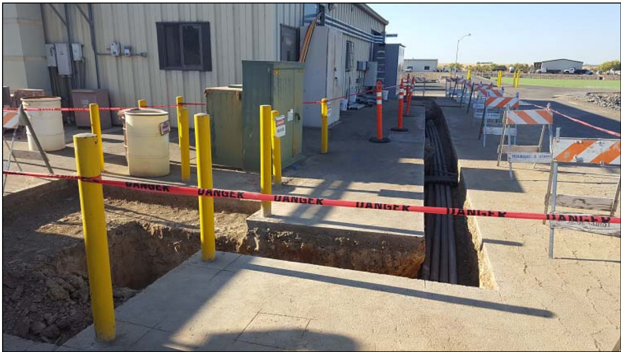
Photo of showing excavation for a future pad for an upgraded SMUD transformer and conduit installations to new electrical switchgear panels.
