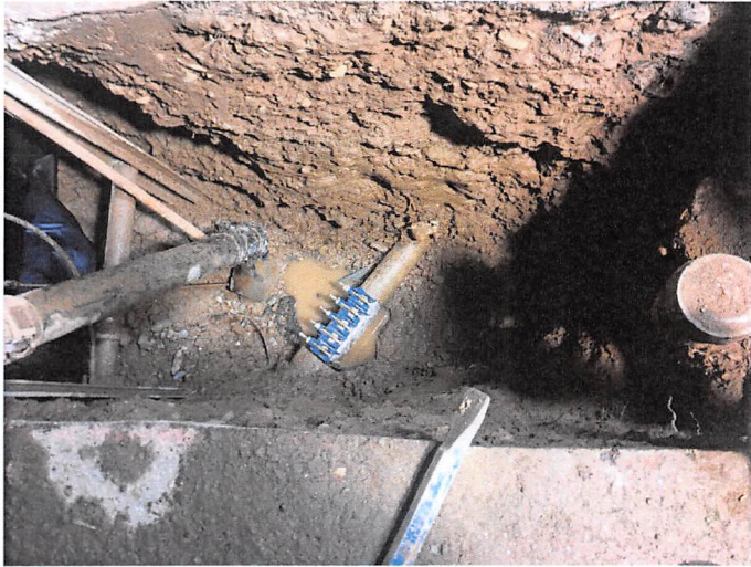
Photo 4: Temporary repair at break dated 12/12/18.
