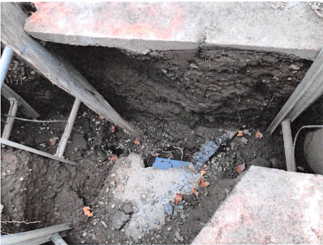
Photo 2: Trench excavation after initial backfill dated 12/13/18. Concrete area in middle of trench is top of thrust block on existing 90 degree bend.
