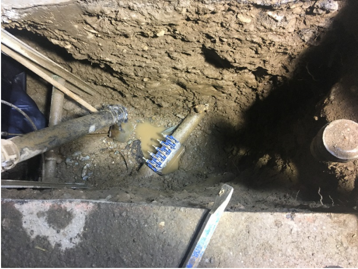
Photo 4: Temporary repair at break dated 12/12/18.
