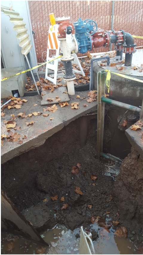
Photo 1: Trench excavation at force main break, illustrating sloughing of trench under existing AC , dated 12/17/18.
