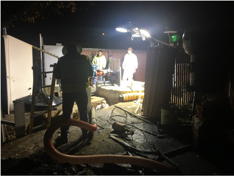
Photo 5: Site when force main was broken dated 12/12/18.
