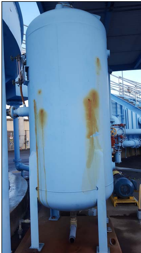
Photo of West DAF saturation tank
