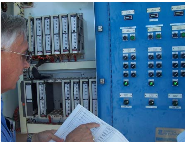
Technician troubleshooting current control panel.
