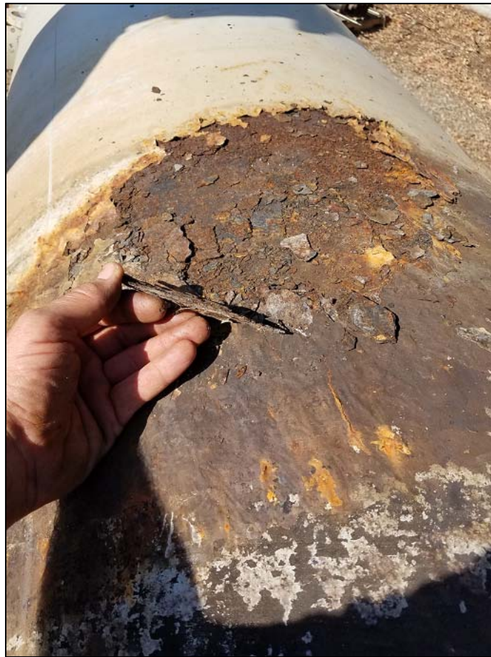
Corrosion of pipe column
