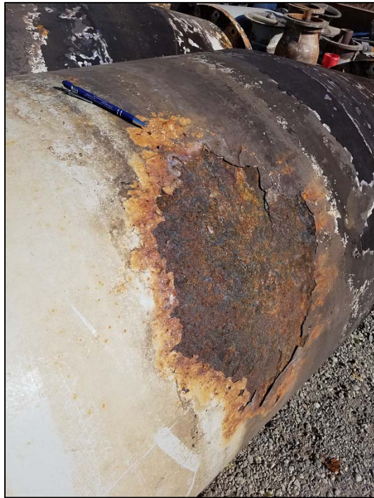
Corrosion of pipe column
