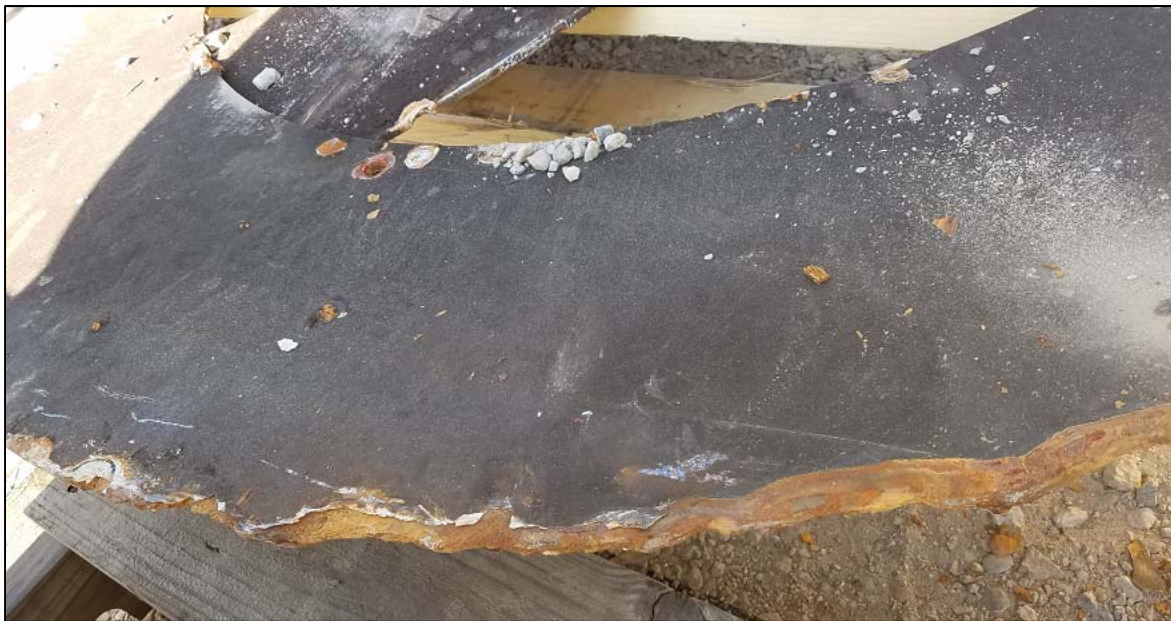
Corrosion of Vortex Plate of pump 2
