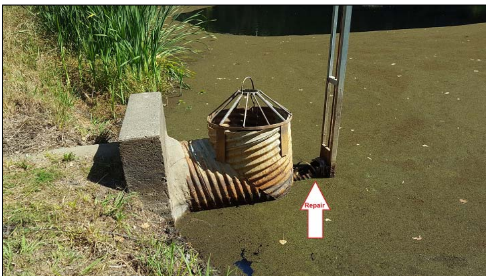
Photo of low flow outlet needing repair at Basin 5
