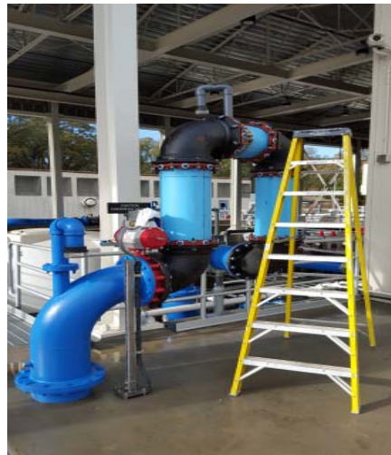
Modified installation of permeate discharge pipe
