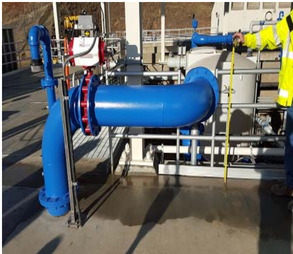
Previous installation of permeate discharge pipe
