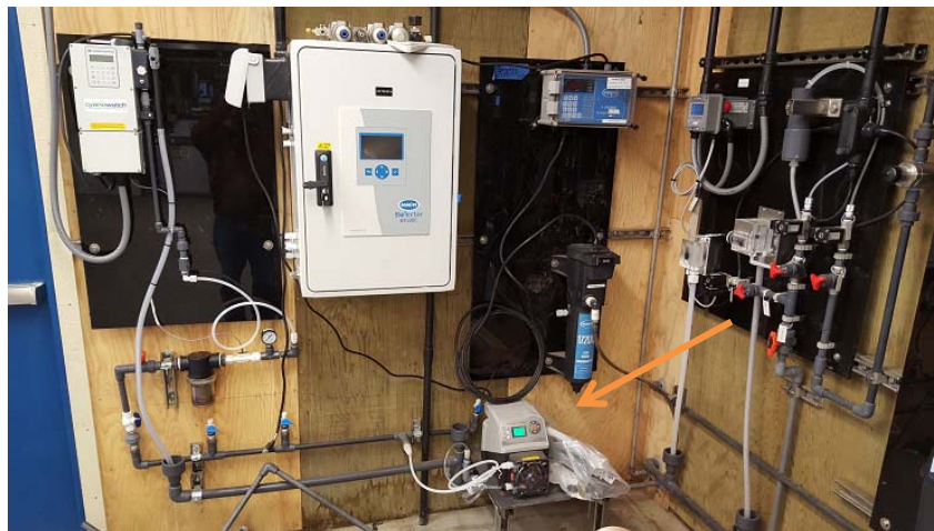
View of some of the water quality equipment; sample pump and lines installed by District Staff
