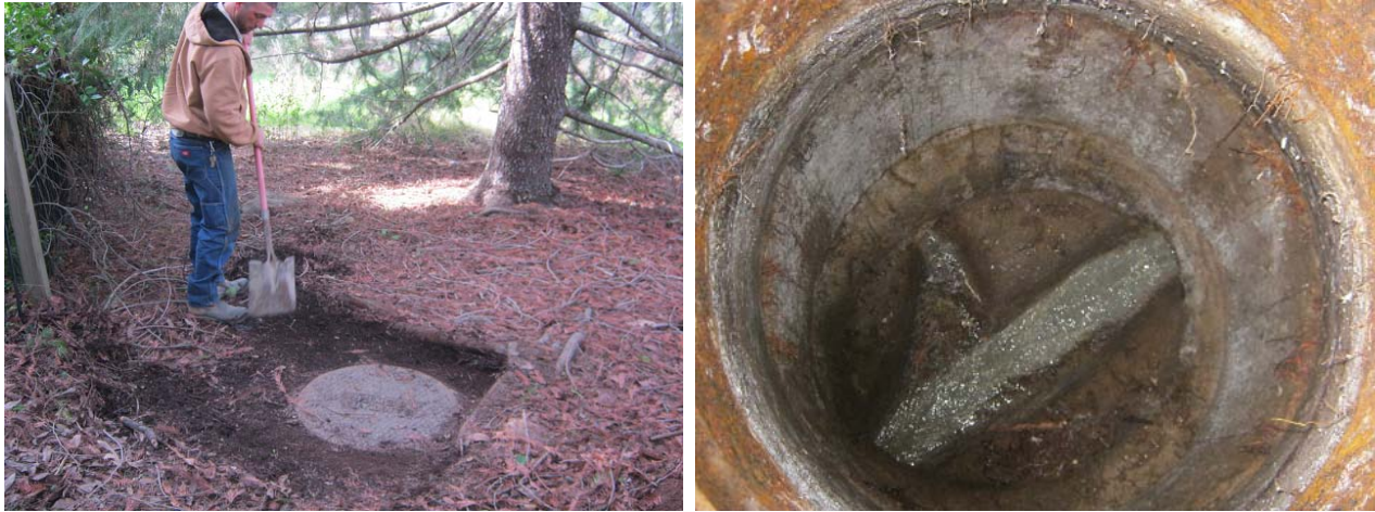
District staff cleaning out around a problematic sewer manhole with minor root intrusion from a Redwood tree. This is in a District easement between 7 Park Terreno and Guadalupe Drive.
