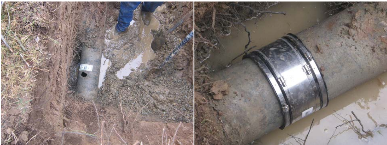
Photos of before and after repair of "Unit 1 sewer lateral B" near Lindero Lane
