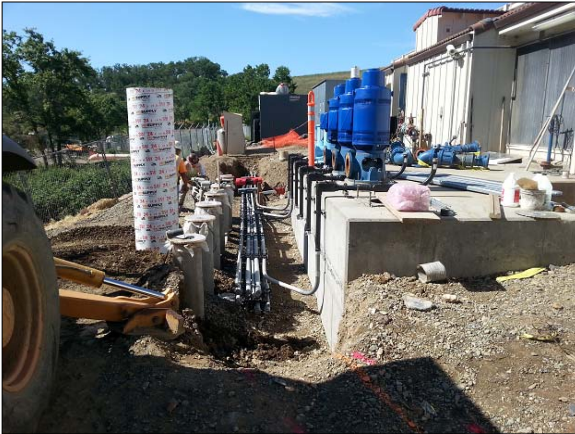
Installation of power and pumps at Effluent Pump station
