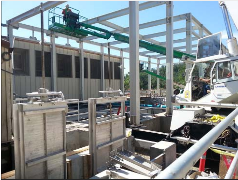
Slide gates at Flash Mix structure in foreground, Erection of Canopy structure background
