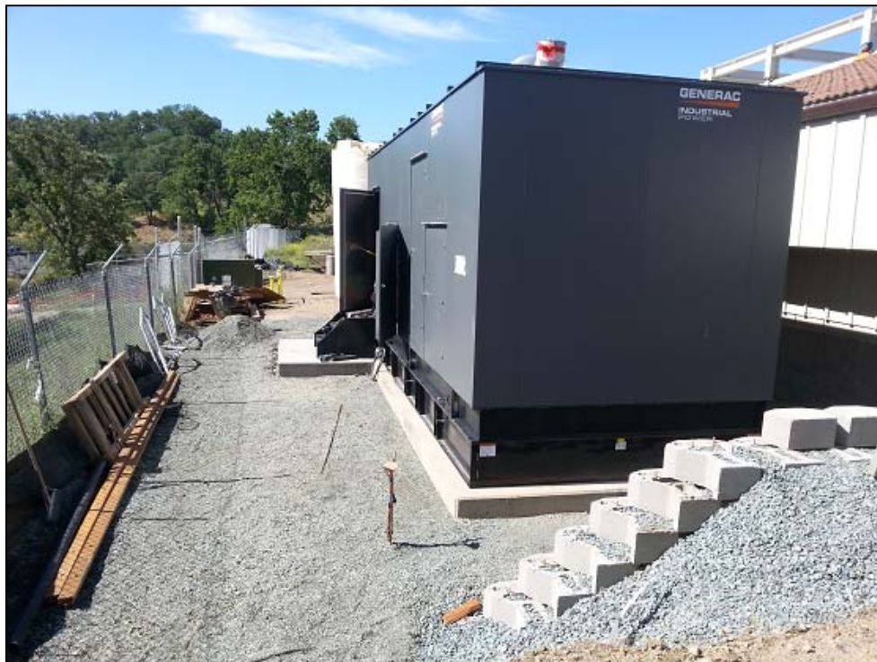
New Generator installed
