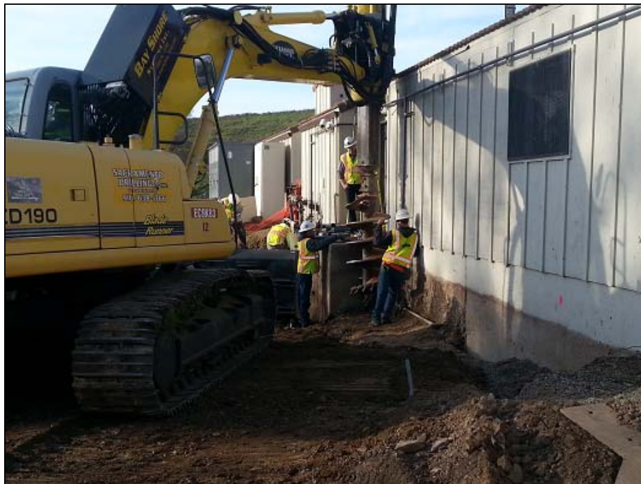
Drilling to install I-beams to shore up building foundation prior to excavating future effluent discharge pump station
