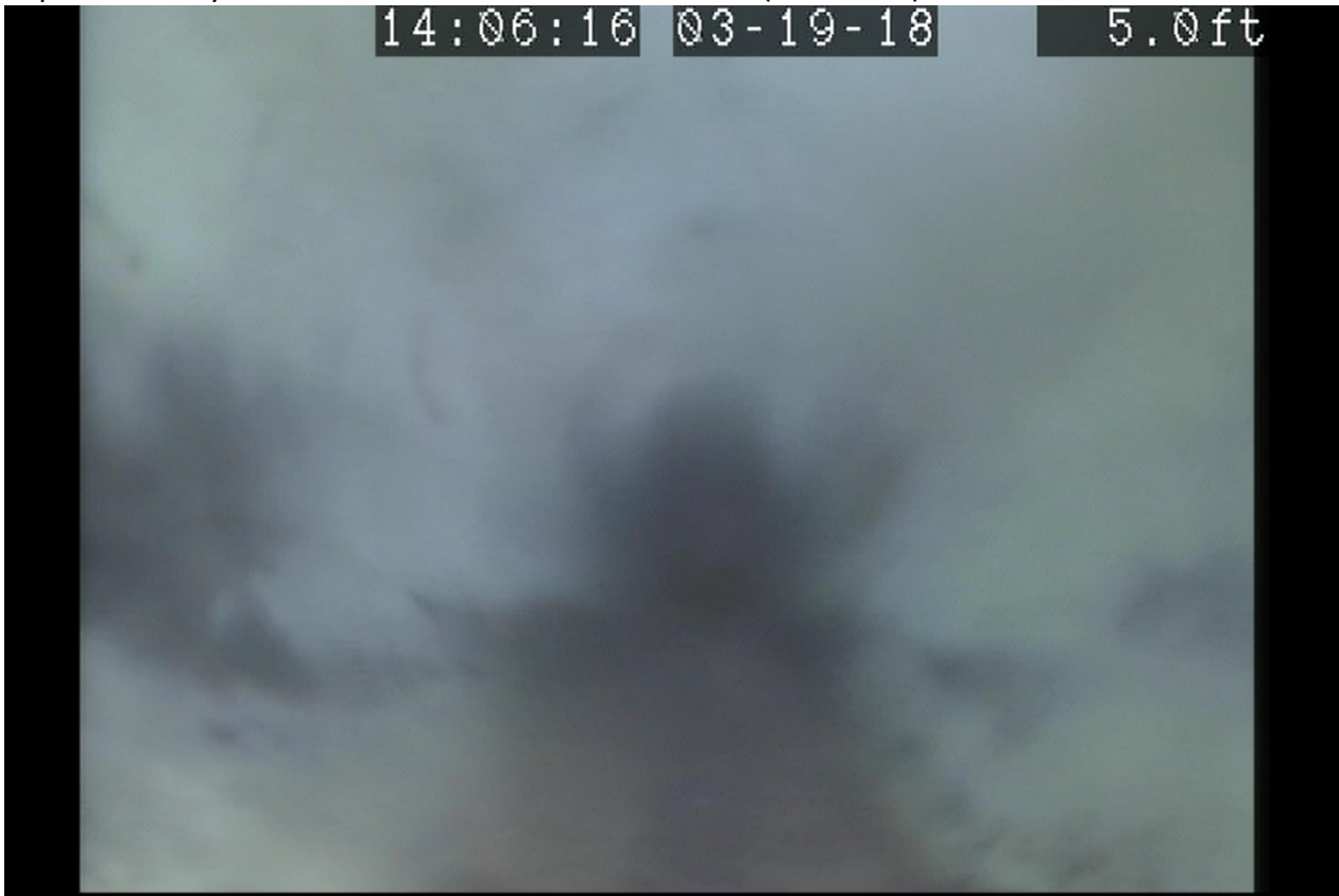
Capture #8: Beyond area of failure toward sewer main (continued)
