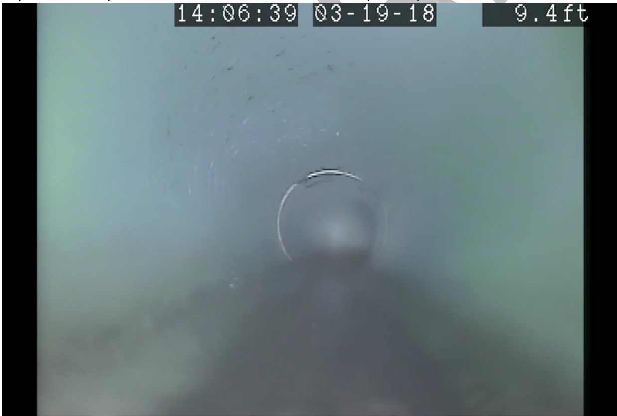
Capture #11: Beyond area of failure toward sewer main (further)
