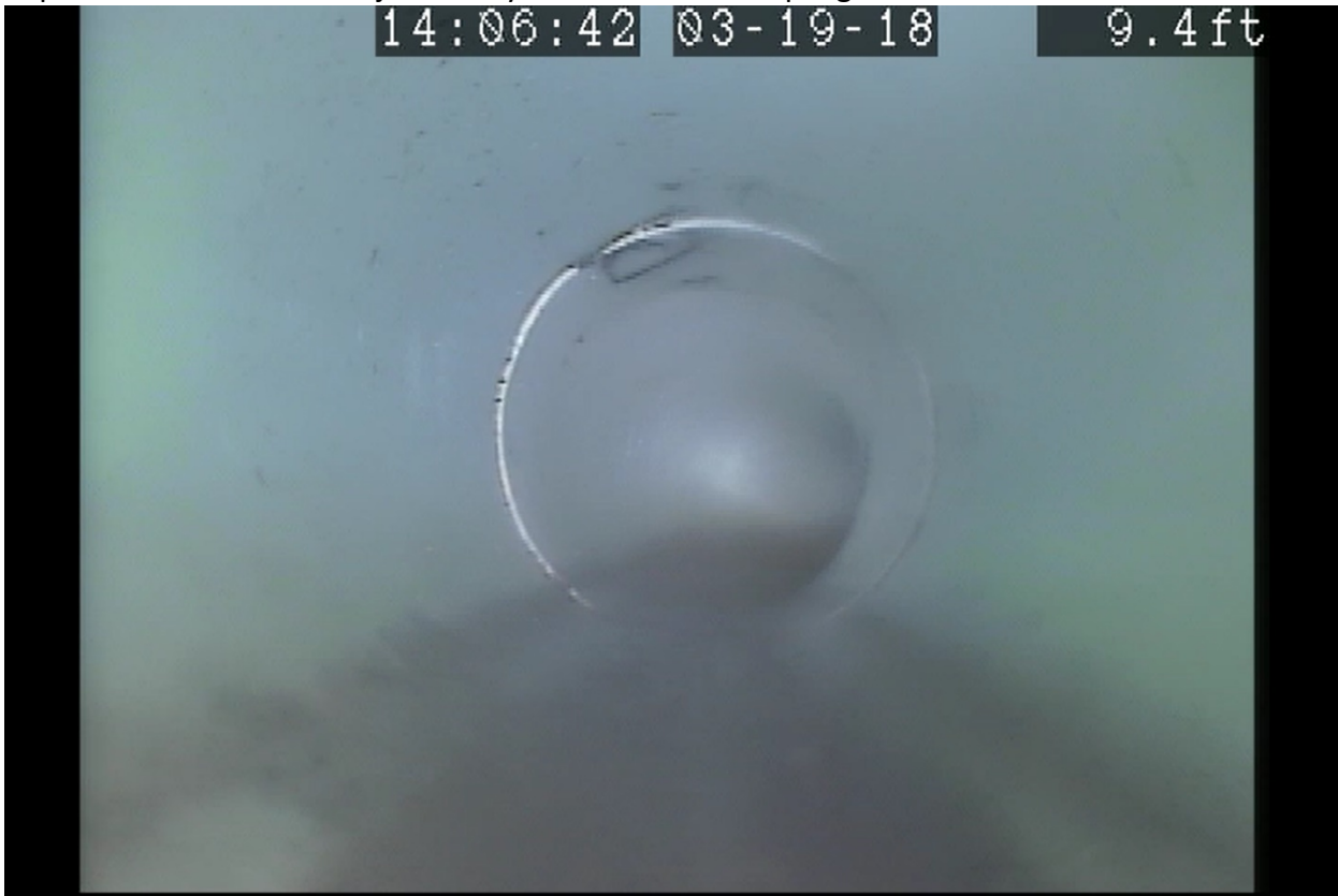
Capture #12: Clear shot of joint likely where flexible coupling to stub exists
