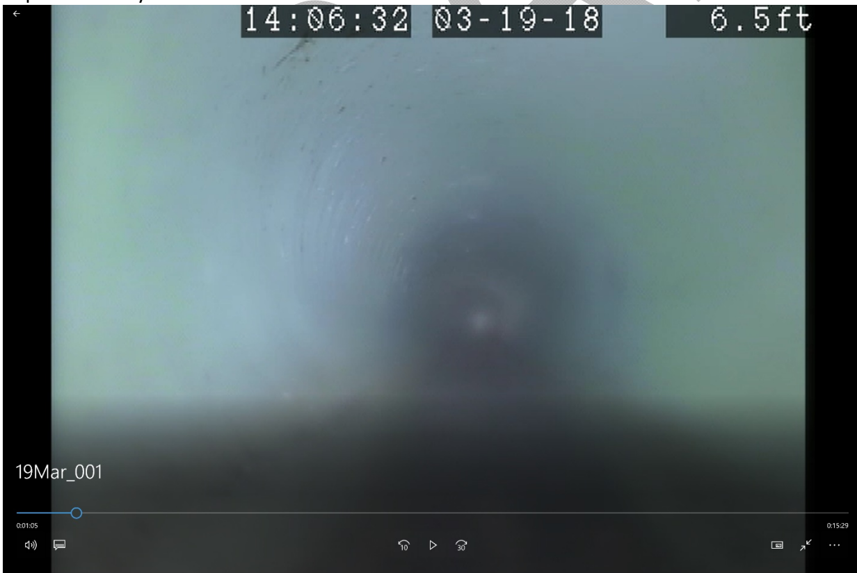
Capture #9: Beyond area of failure toward sewer main
