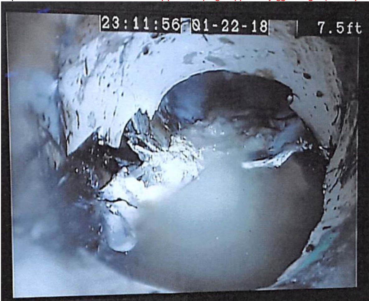
Capture #6: Shot of failure area taken by prior scoping – apparent jagged edges (January 22, 2018)
