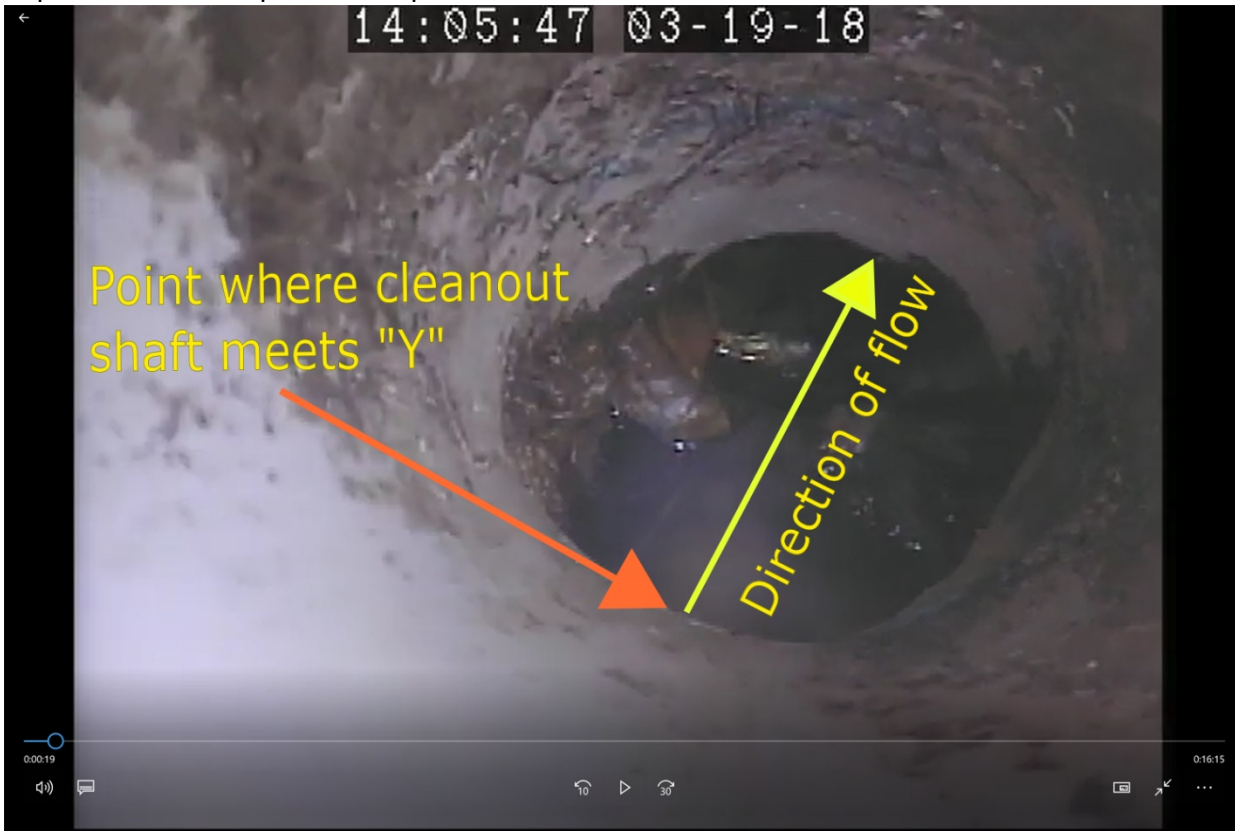
Capture #4B: Same photo of Capture 4A with annotation – Area of failure
