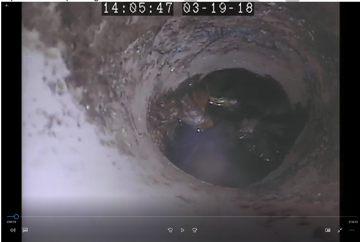
Capture #4A: Scope being lowered down shaft of cleanout at cleanout "Y"
