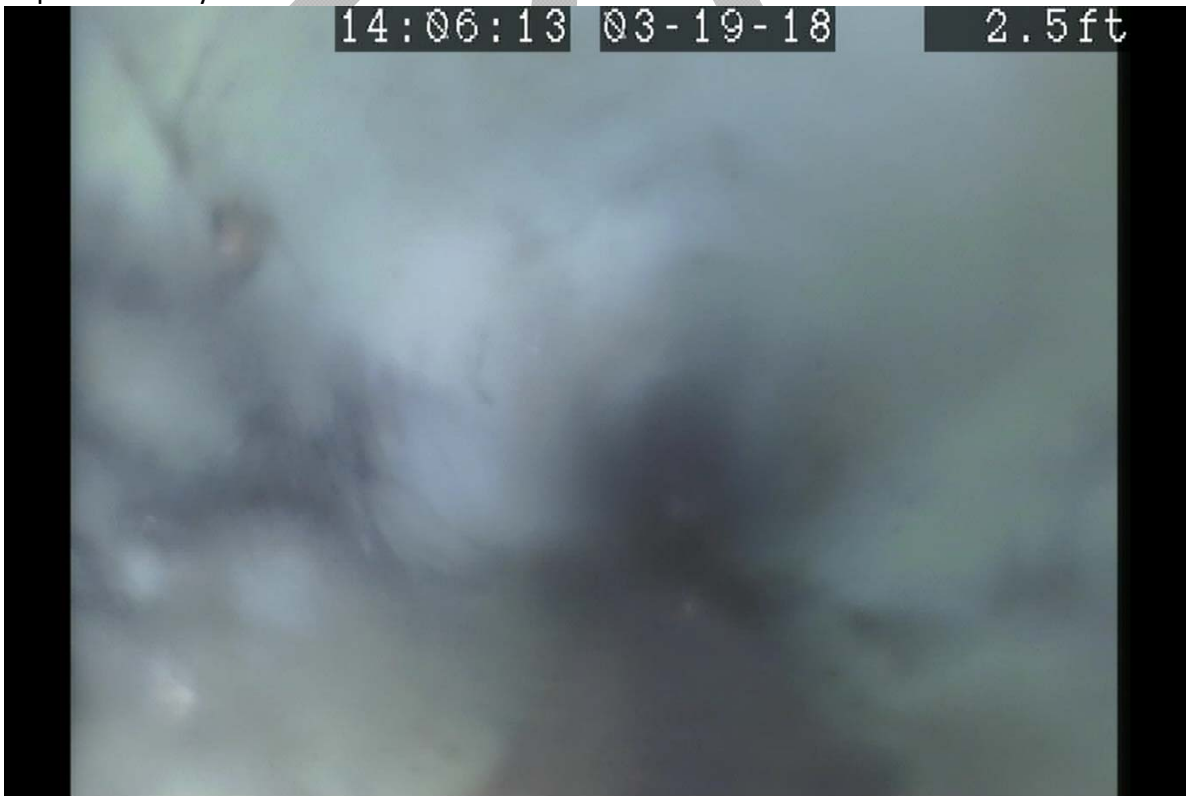
Capture #7: Beyond area of failure toward sewer main
