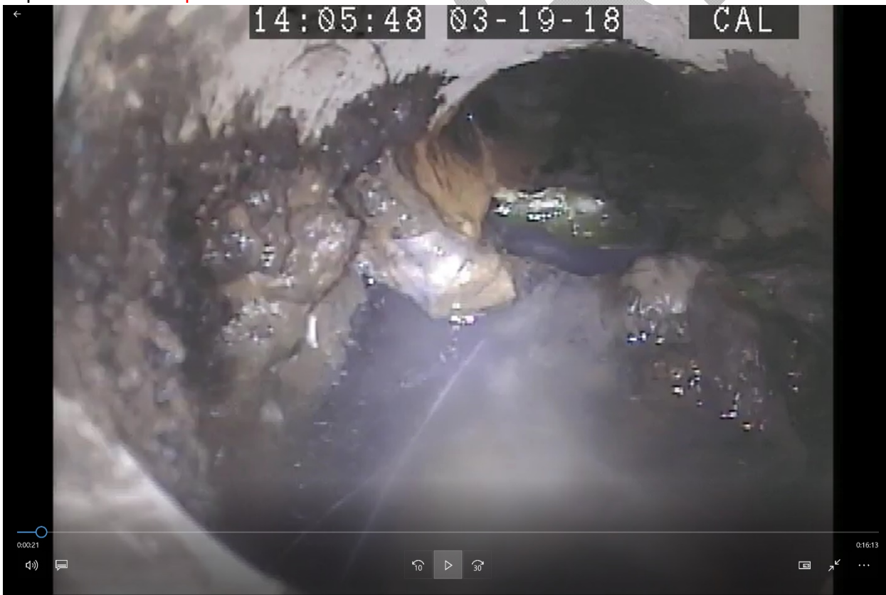
Capture #5: Close-up of area of failure
