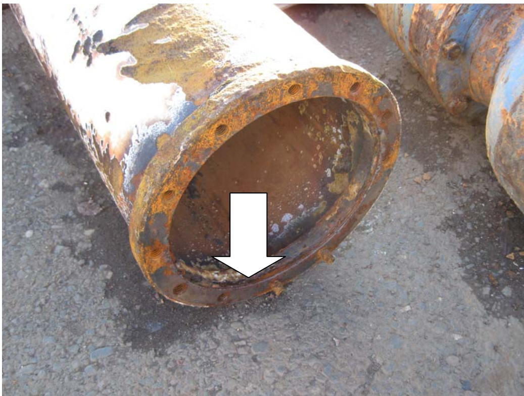
Figure 2 - Adapter from pump to column rabbet corroded and needs to be cut off and replaced
