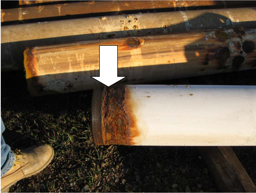
Figure 7 - Focused corrosion causing some pipe column sections to be replaced
