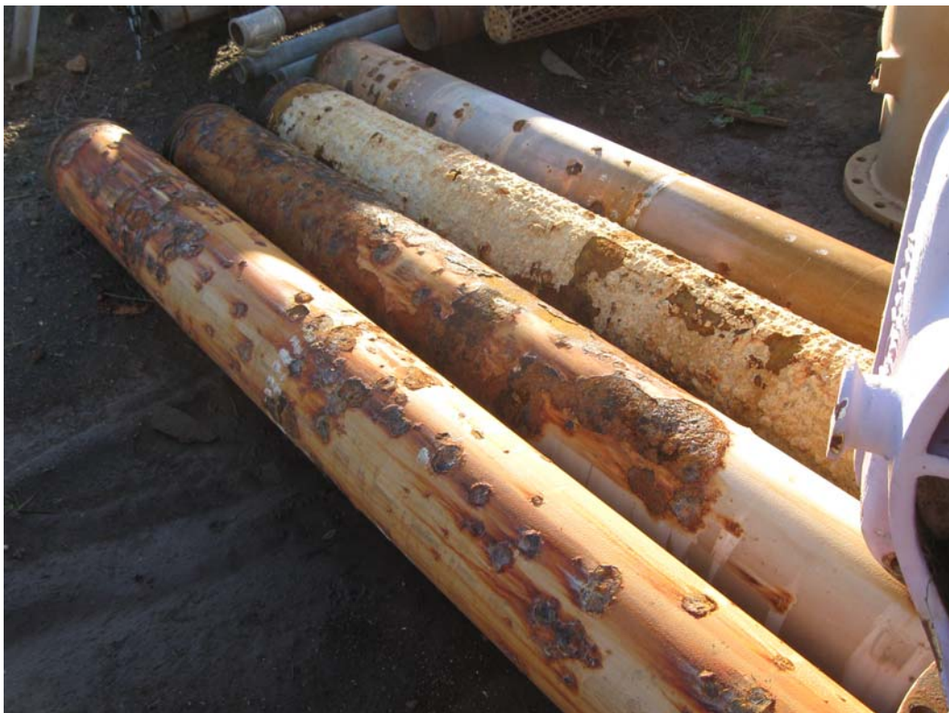
Figure 6 - Focused corrosion causing some pipe column sections to be replaced
