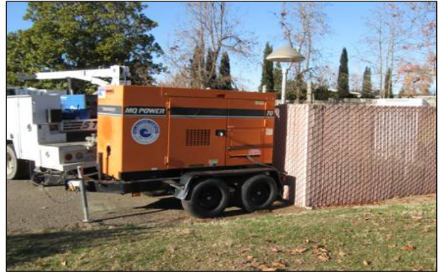
Temporary standby generator at Cantova Lift Station
