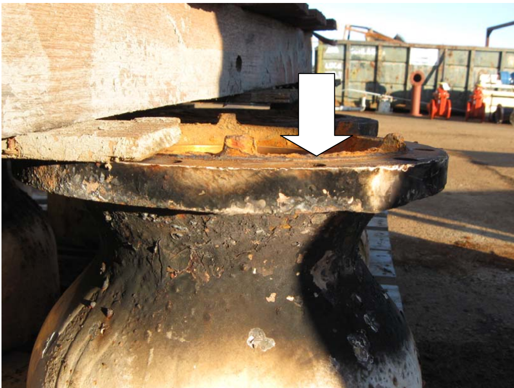
Figure 4 - Bad rabbet on bowl due to corrosion ~1/8" thick
