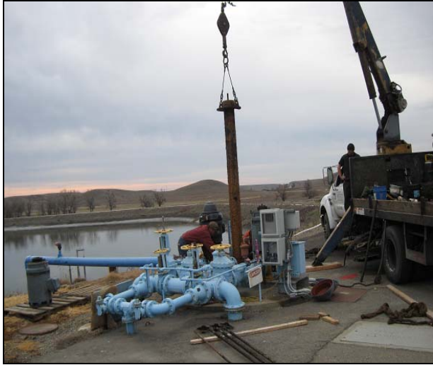
Kirby Pump pulling one of the Tertiary pumps covered by corrosion.
