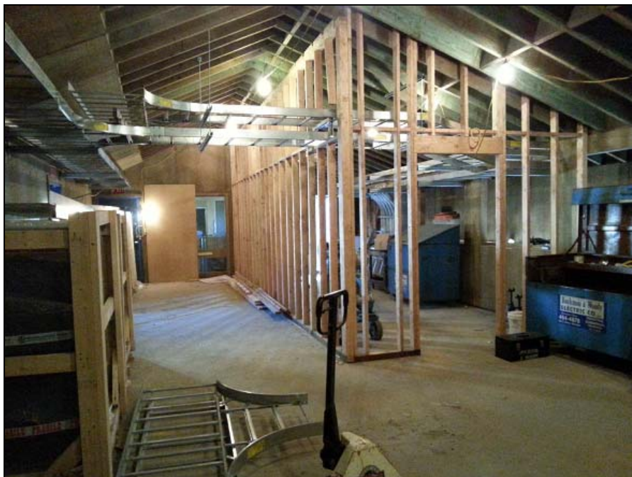
Framing and cable tray installation in future membrane equipment and control rooms.
