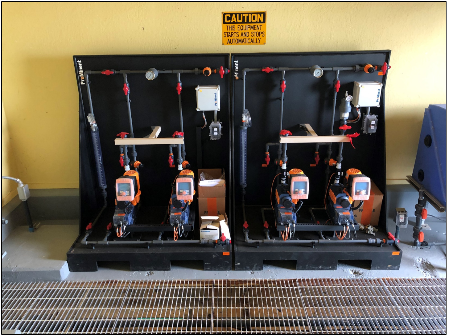
Chemical feed skids placed in chemical feed room of Wastewater Reclamation plant
