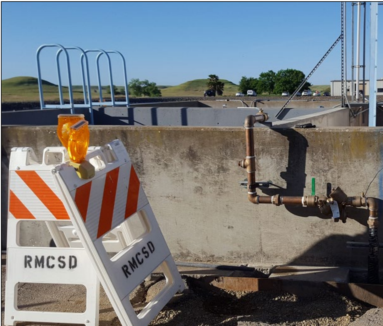
Installation of a water fill line for dilution of new chemical tanks
