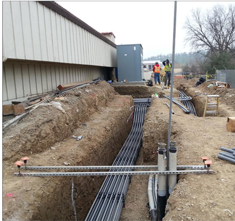
Electrical Conduits for new power feed
