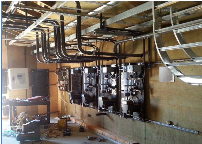
Water quality monitoring equipments installations
