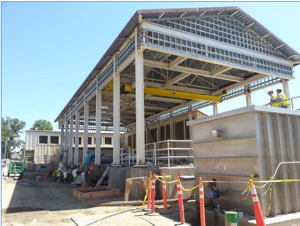
Membrane area canopy structure with Plate Settler in foreground
