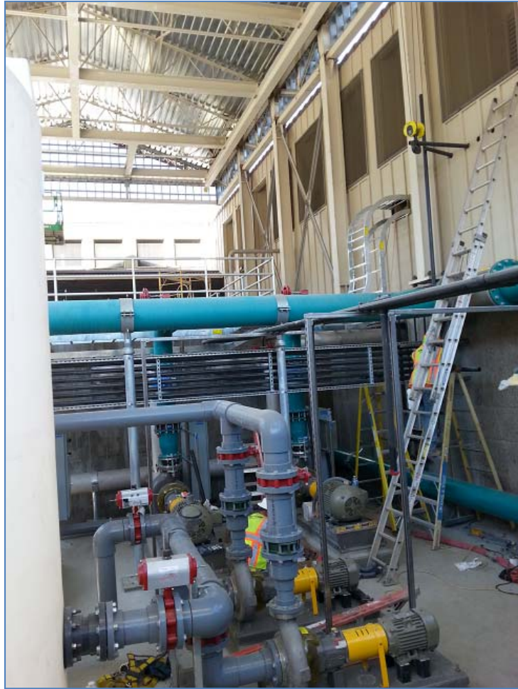
View of CIP pumps in foreground, Permeate pumps in background and wiring runs
