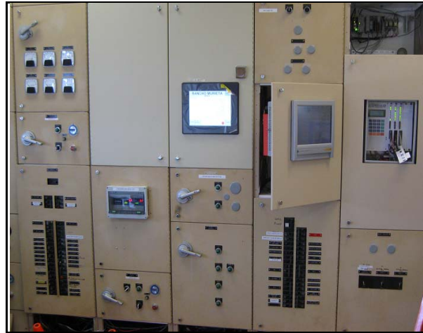
Preview of new panels with HMI (Human machine interface)
