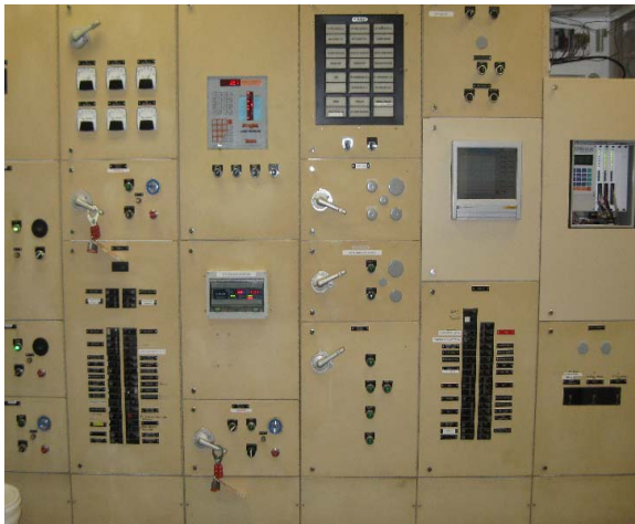
Old view of WW Plant RTU(remote terminal unit) #1
