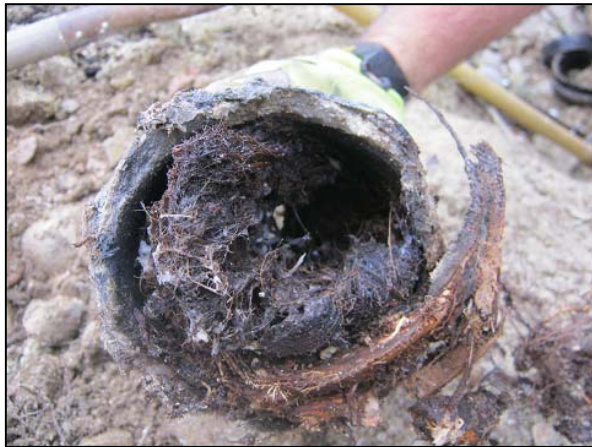
Service line with tree roots in it, replaced by staff.
