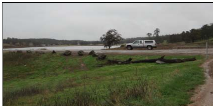
Photo of debris placed near PTF gate at Clementia to discourage driving on dam.
