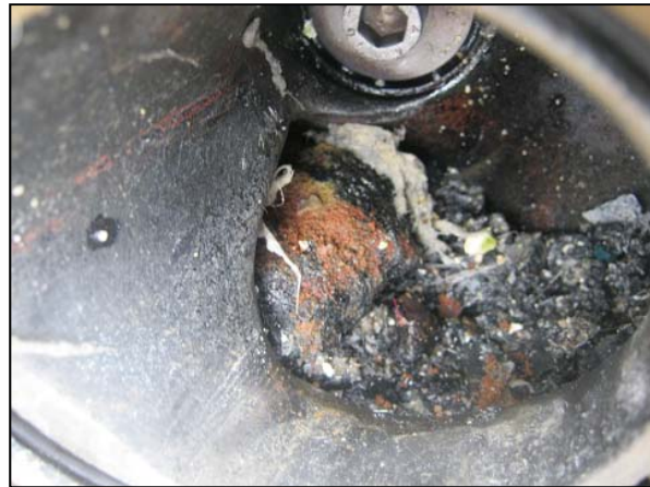
Debris lodged in suction of Crest sewer lift station pump.
