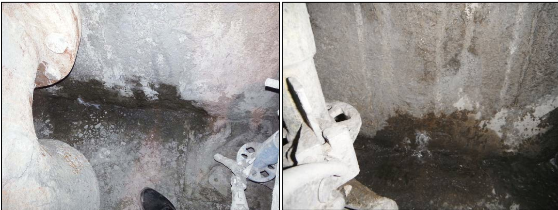
Photos showing water intrusion into wet wells
